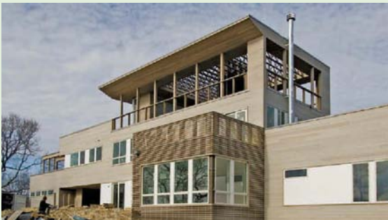
Exterior Finish: Contractor Harland Frazier and his workers spent several months finishing the home's interior and exterior.
