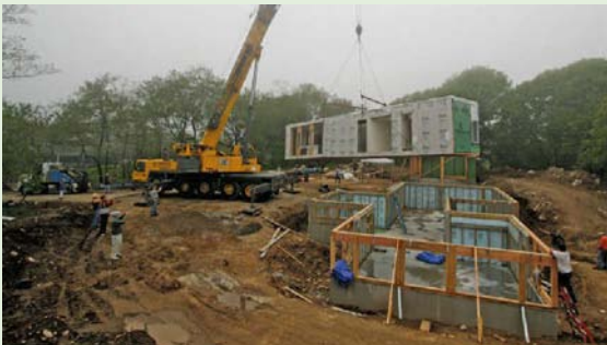
First Box: After arriving on the island by ferry, the boxes were set on the foundation by a crane.
