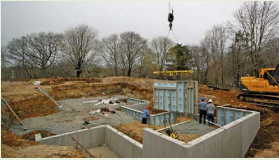
Foundation Down: The house's cement foundation is also modular, and was installed by Superior Walls of Pennsylvania.
