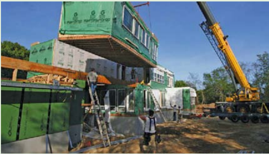
Crunch Time: Once the boxes were set in place, the on-site workers spent two days connecting them to each other and to the foundation.
